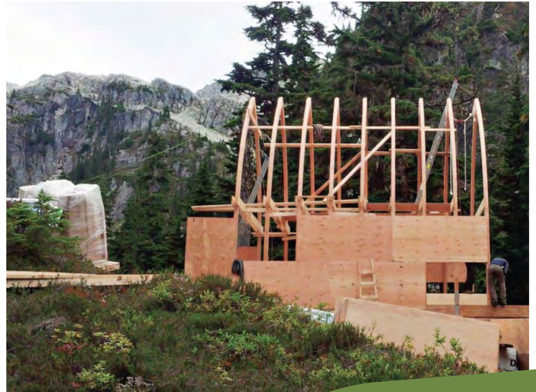
FRAMING UP A DREAM. SCANLON DRIVES A FEW NAILS HOME. PHOTO: ED ZENGER
